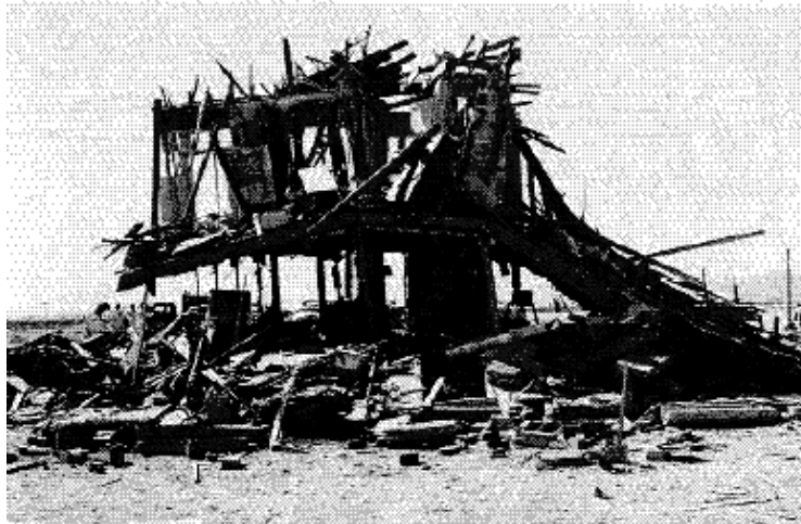
Figure 8-2 Wood Frame Building After Long Duration Blast Load with 34 KPa (5 psi) Peak Overpressure
