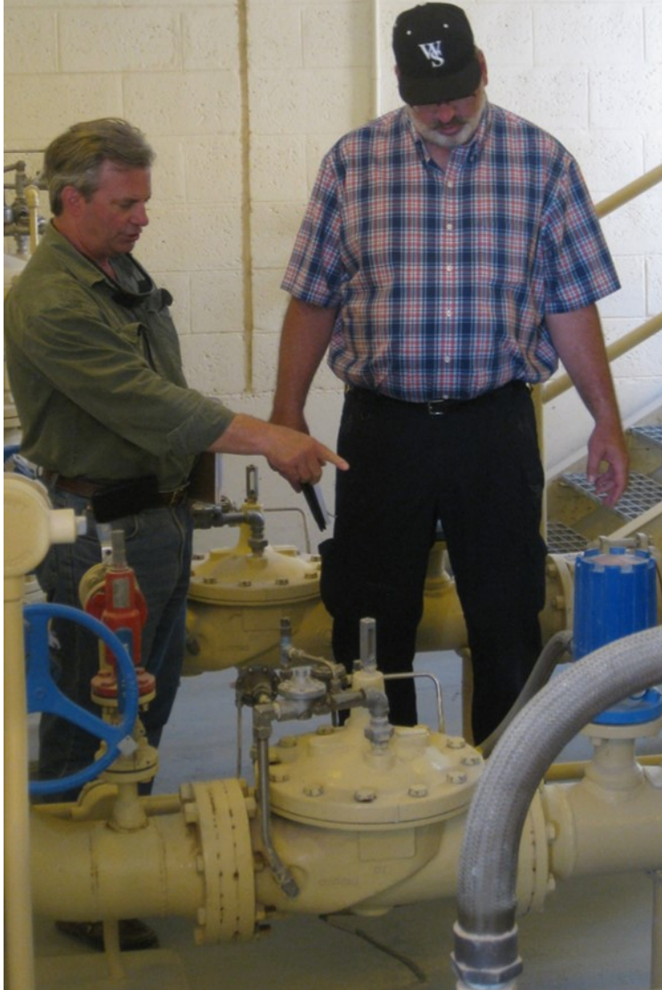
Jim Howell, DoD OIG (left) and Rick Bussard, POL-MCX, Electrical Engineer (right) discuss the operation of an automatic control valve in a fuel pumphouse at AUAB. Photo by Greg Etter.
