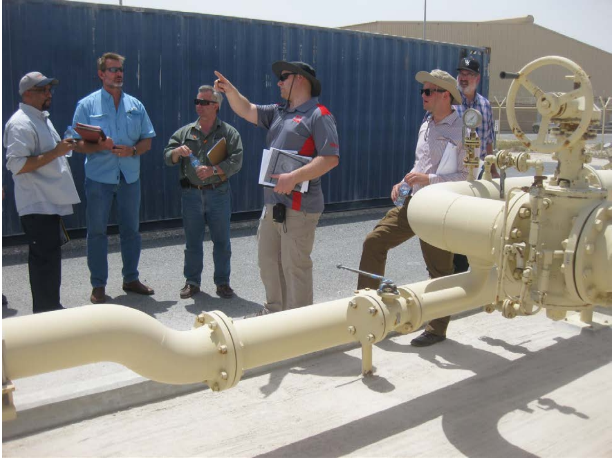
Eric Bausch, POL-MCX, Civil Engineer explains the pigging launchers and receivers located at AUAB. Left to right: Chris Wells, AUAB fuels maintenance; Nicolaas Degreef, DLA; Jim Howell, DoD OIG; Eric Bausch, POL-MCX, Civil Engineer; Dustin Scheuffele, POL-MCX, Mechanical Engineer and Rick Bussard, POL-MCX, Electrical Engineer. Photo by Greg Etter.
