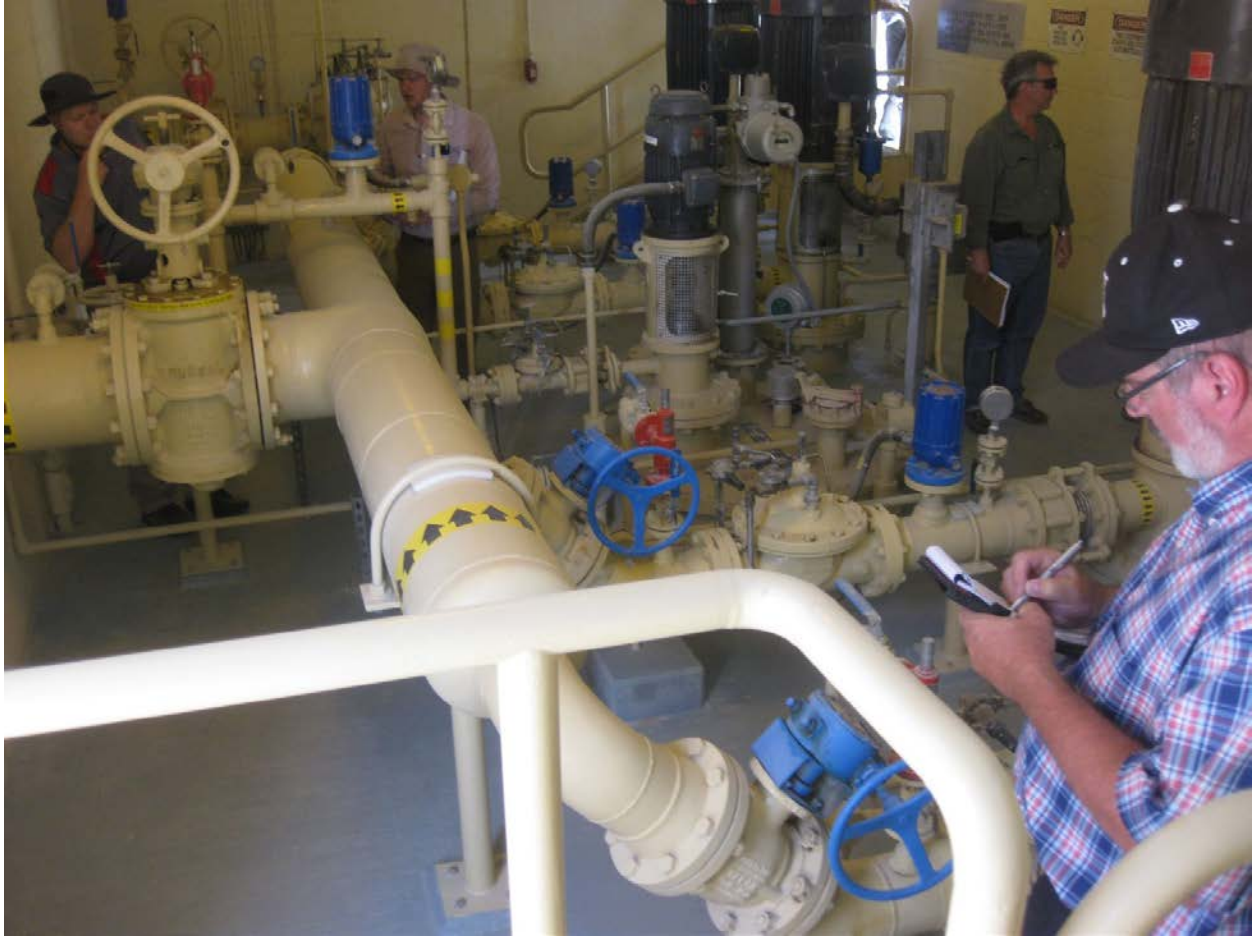
POL-MCX team inspect a fuel pumphouse at AUAB. Left to right: Eric Bausch, POL-MCX, Civil Engineer; Dustin Scheuffele, POL-MCX, Mechanical Engineer; Jim Howell, DoD OIG and Rick Bussard, POL-MCX, Electrical Engineer. Photo by Greg Etter.
