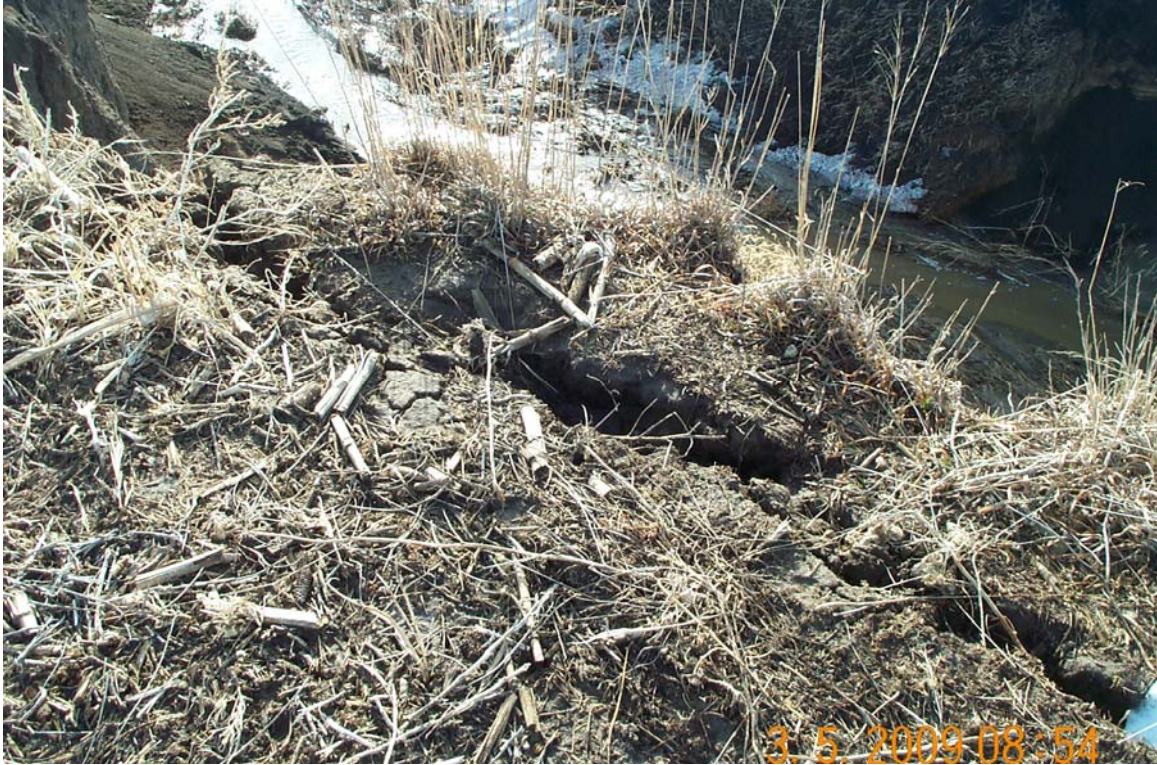
#9 Chunk of stream bank about to fall in
