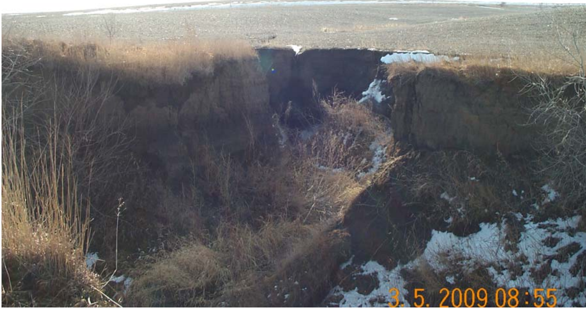
#11 Looking Southeast -- scour hole along bank line
