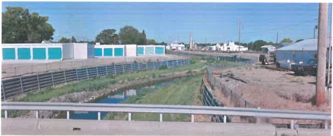
Figure 79. View of South 5 th Avenue Bridge, looking upstream, shows how Mud Creek is confined
