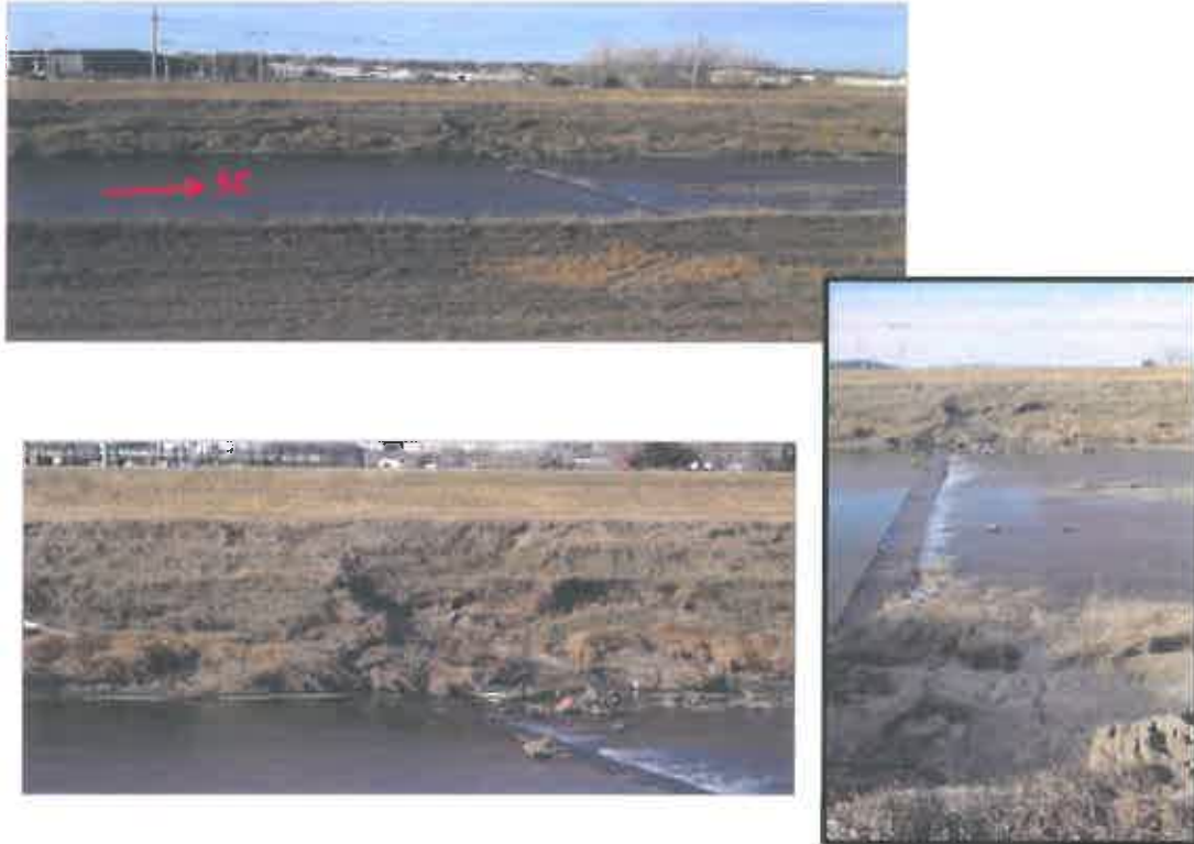
Figure 45. Typical conditions found along Salt Creek in Lincoln, Nebraska
