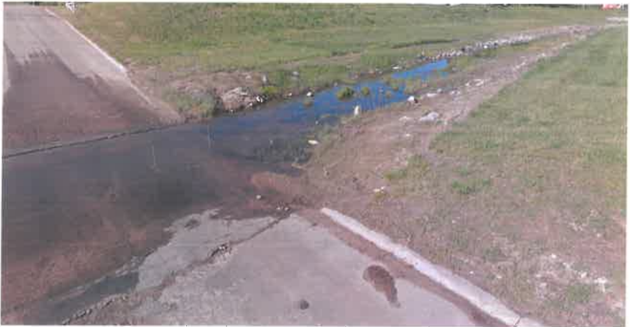
Figure 74. View of the South 15 th Avenue Bridge, looking upstream, shows Mud Creek flowing over the road during low flow periods
